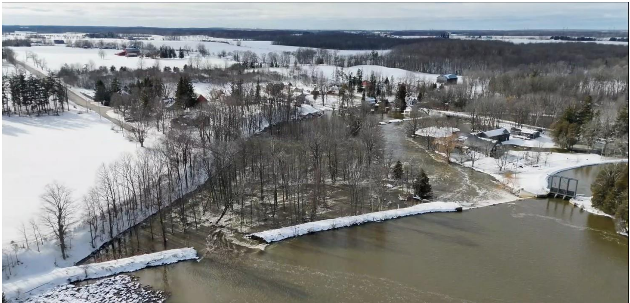
An Aerial Overview of the Privately Owned Flood Control Structure Breach - March 15, 2026
