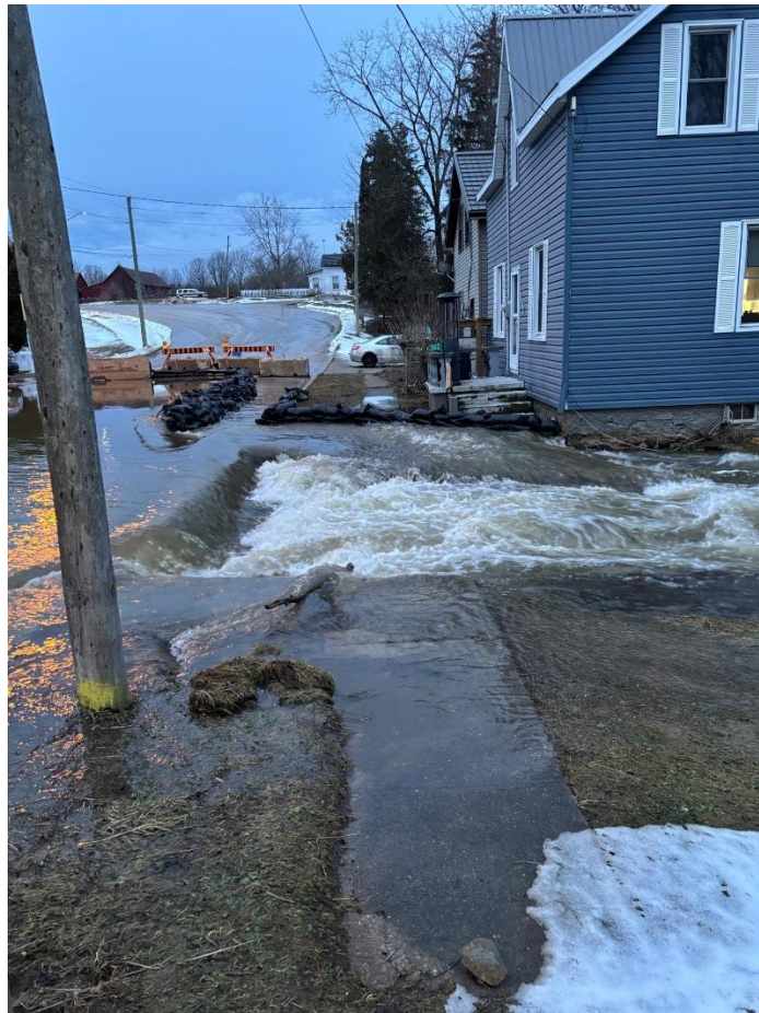
Flooding Observed Across Bruce Road 15 - March 16, 2026
