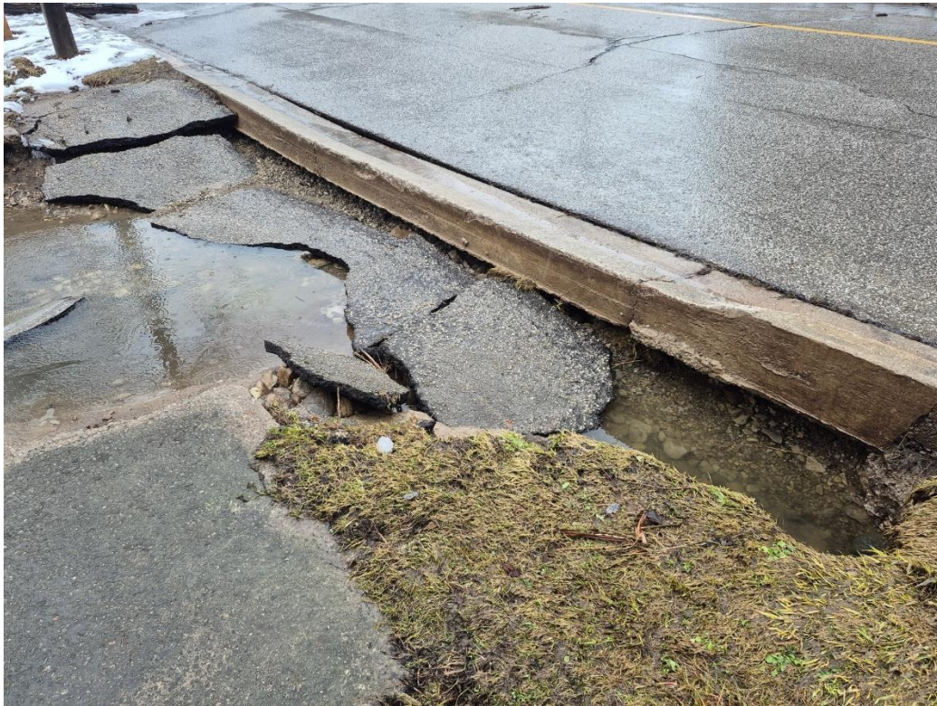
Damage to Bruce Road 15 - March 21, 2026
