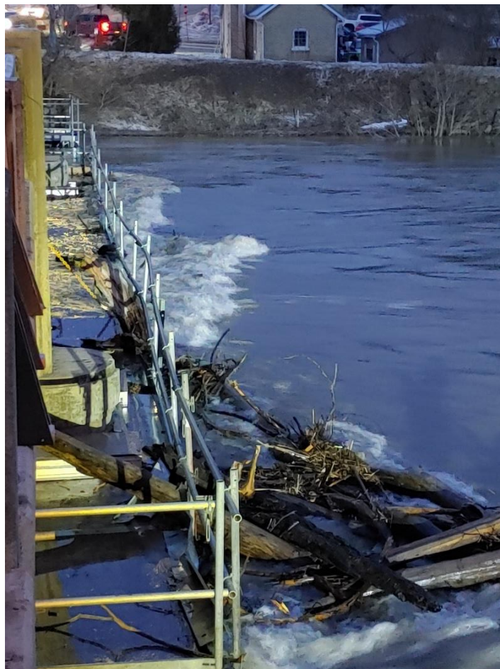
Photographs of Flooding & Debris at Durham Street Bridge, March 17-18, 2025
