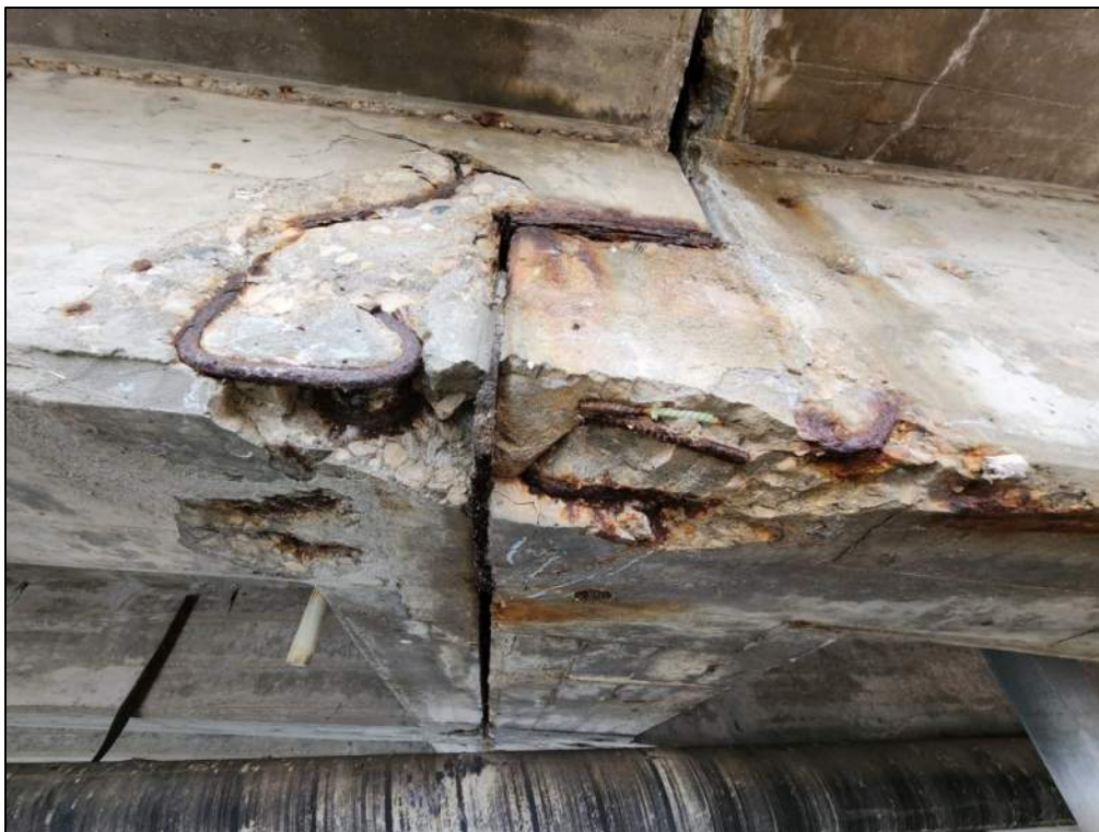
Photo P65 – Soffit between Pier 2 to Pier 3 (delamination, spall with exposed corroded rebar and rust staining at drop in span joint- severe rust on bearing plates; evidence of leakage)
