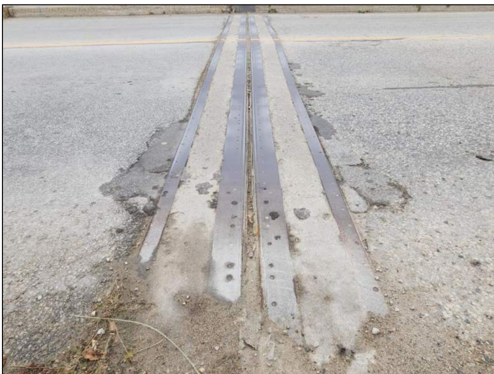
Photo P12 – East Expansion Joint (strip seal joint; light rusting on the steel armoring angles; seals covered with dirt and debris; cracks, spalls and scaling at concrete end dams- gap dimensions 45mm throughout)
