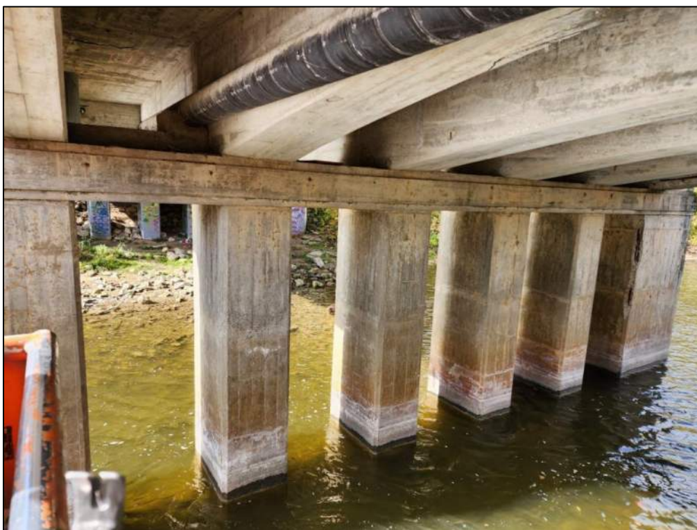
Photo P46 – Pier 2 – East Face (spall, delamination and hairline to narrow efflorescence stained cracks, light pattern cracks)
