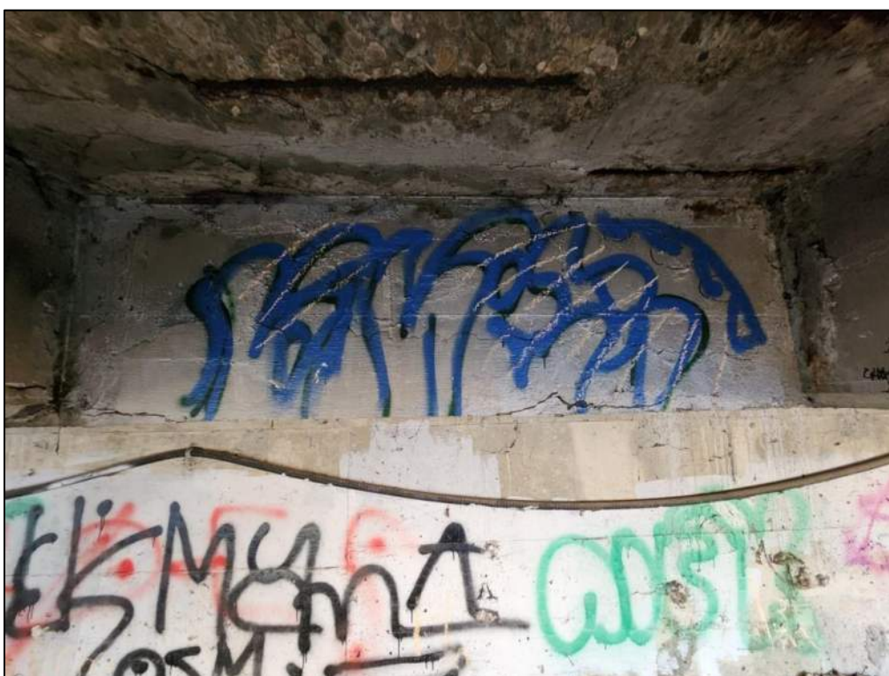
Photo P84 – West Abutment Diaphragm (delamination)
