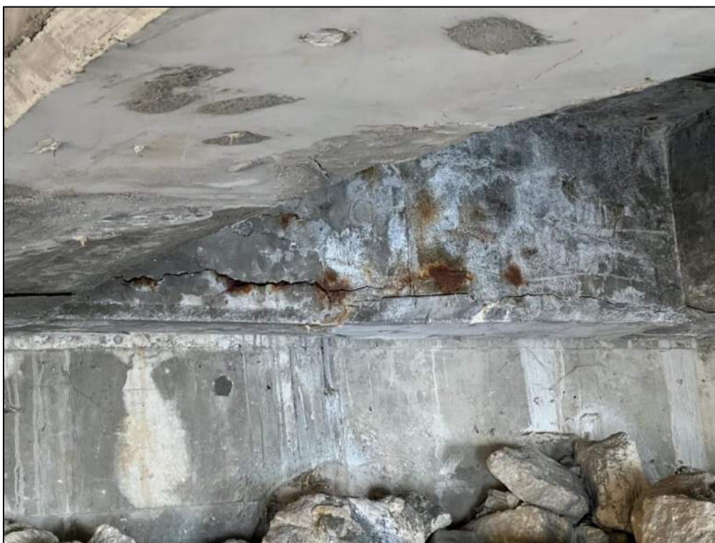
Photo P86 – East Abutment Diaphragm (delamination, rust stains)
