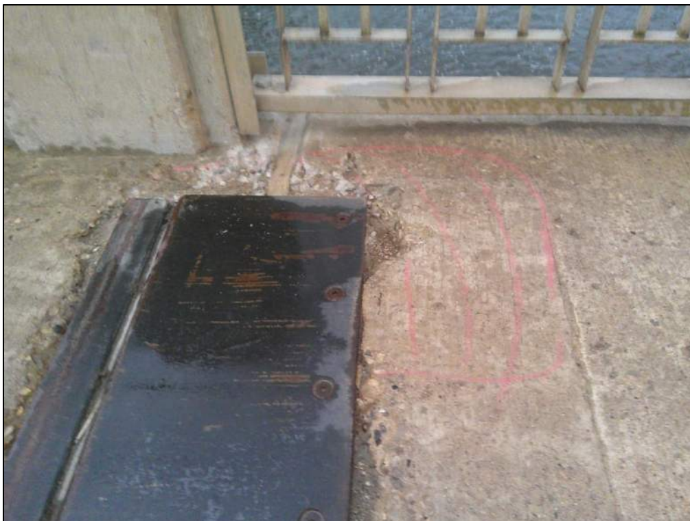
Photo P17 – North Sidewalk delamination and spall near west intermediate expansion joint)
