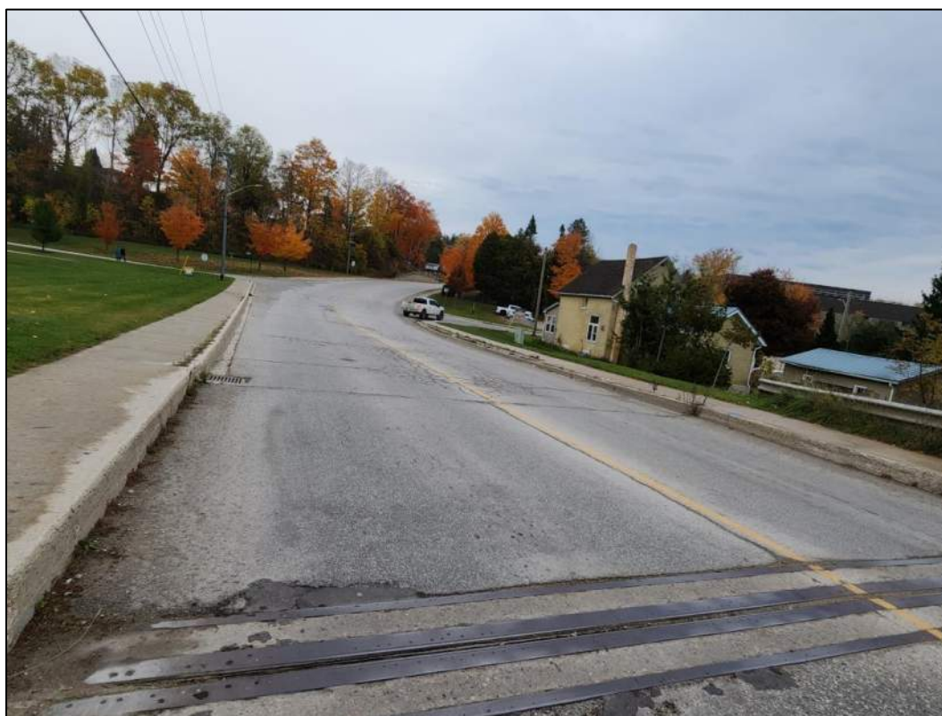
Photo P6 – East Approach Wearing Surface (good condition – unsealed cracks, patches and light ravelling)
