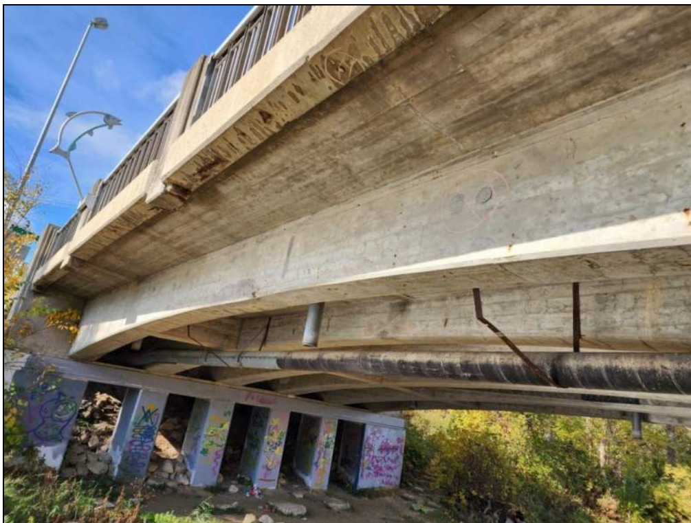
Photo P61 – Soffit between Pier 1 to Pier 2 (spalls with exposed corroded rebar, delamination and patched areas) and Girders (delaminations and patched area)
