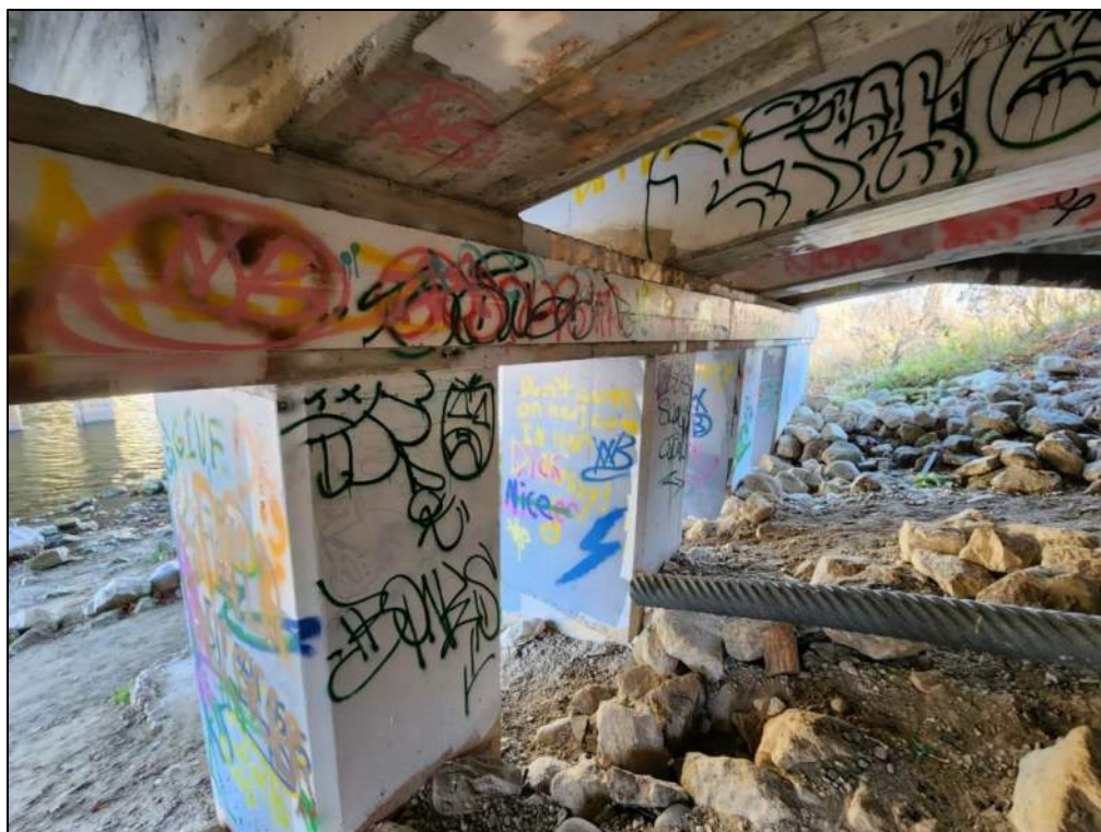
Photo P39 – Pier 1 – West Face (spalls with exposed corroded rebar)
