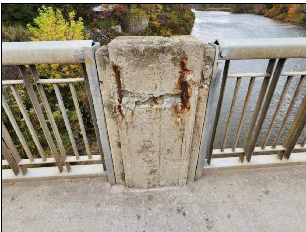
Photo P24 – South Concrete Post (spalls with exposed corroded rebar)
