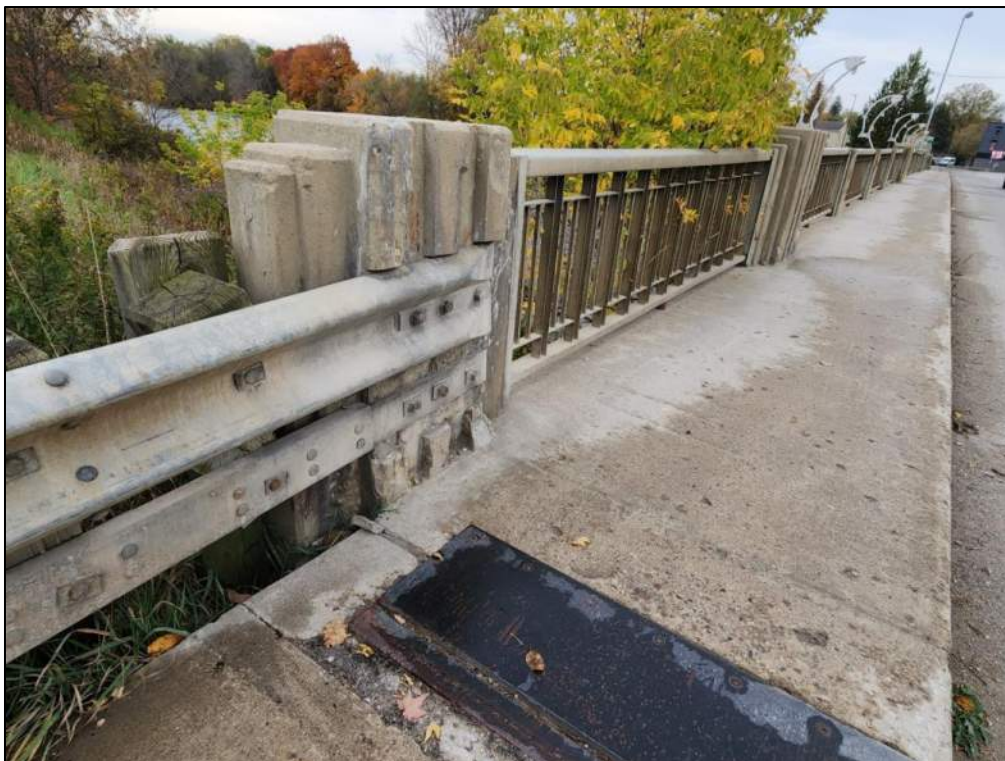
Photo P19 – South Sidewalk (fair condition – crack, delaminations and shallow pop-outs) and Steel Handrail (fair to good condition – bent railings)
