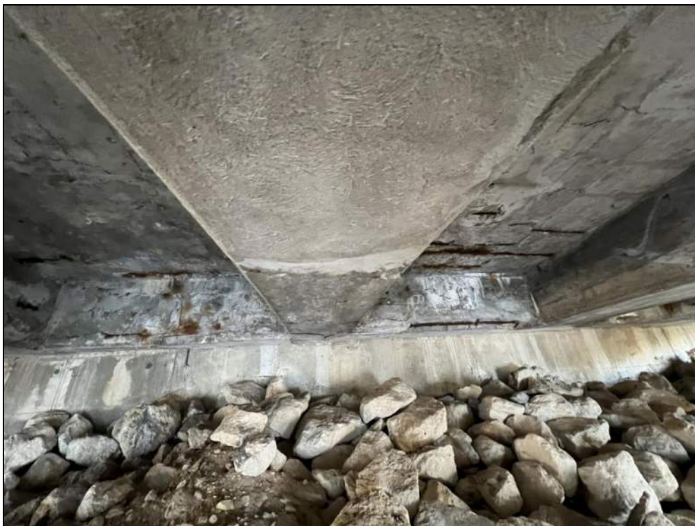
Photo P85 – East Abutment Diaphragm (crack, spall with exposed corroded rebar and delamination, rust stains)
