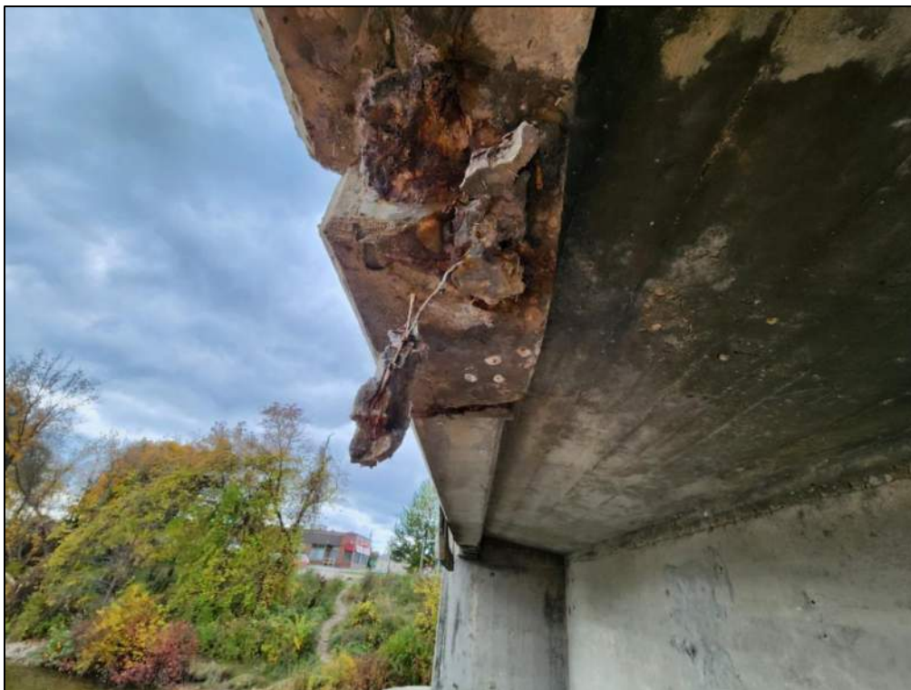
Photo P67 – Soffit between Pier 2 to Pier 3 (spall with exposed corroded rebar and delamination at bottom face of post)
