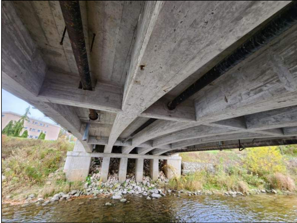
Photo P69 – Soffit between Pier 3 to Pier 4 (spalls with exposed rebar, delaminations and patched areas) and Girder (delaminations and patched areas)
