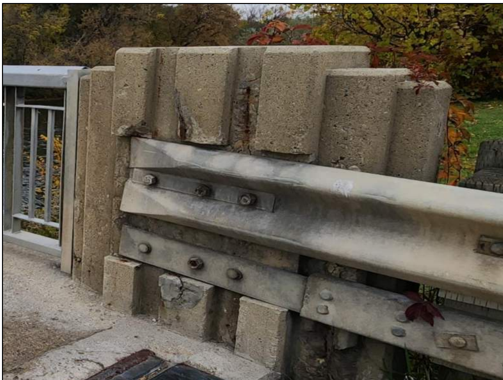
Photo P27 – North-East End post (spalls with exposed corroded rebar, patches)
