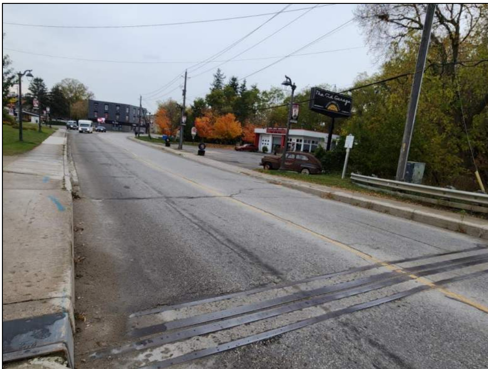
Photo P7 – West Approach Wearing Surface (good condition – sealed/unsealed cracks and light ravelling)
