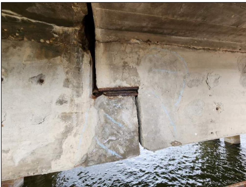
Photo P64 – Soffit between Pier 2 to Pier 3 (delamination, spall and rust staining at drop in span joint-severe rust on bearing plates; evidence of leakage)
