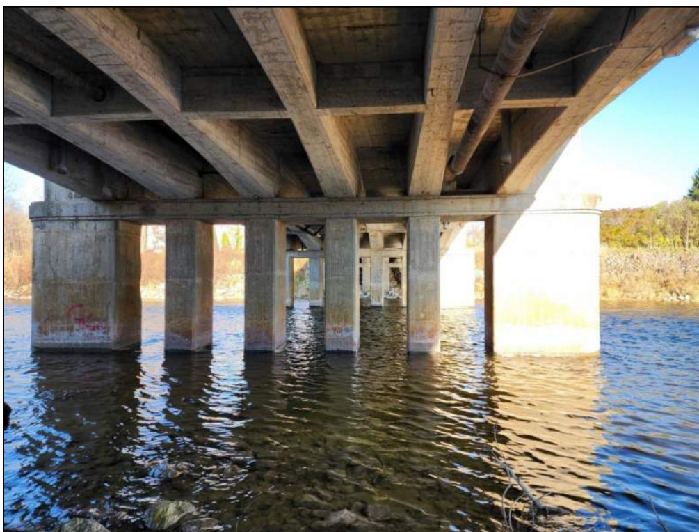
Photo P44 – Pier 2 – West Face (crack and light scaling)
