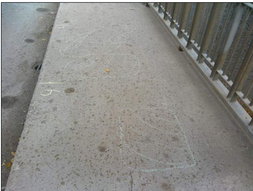
Photo P20 – South Sidewalk (delaminations)
