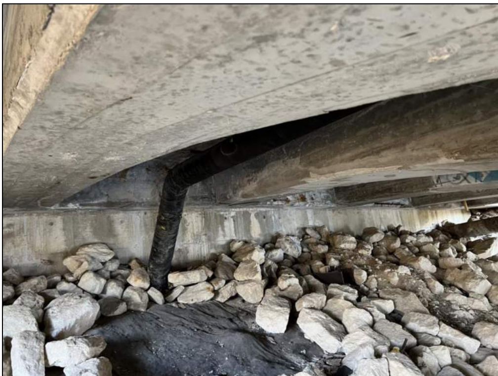
Photo P38 – East Abutment (good condition) and Embankment (fair to good condition – erosion, loss of rock protection)
