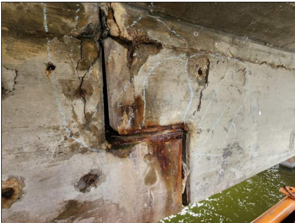
Photo P63 – Soffit between Pier 2 to Pier 3 (delamination, spall and rust staining at drop in span joint-severe rust on bearing plates; evidence of leakage)
