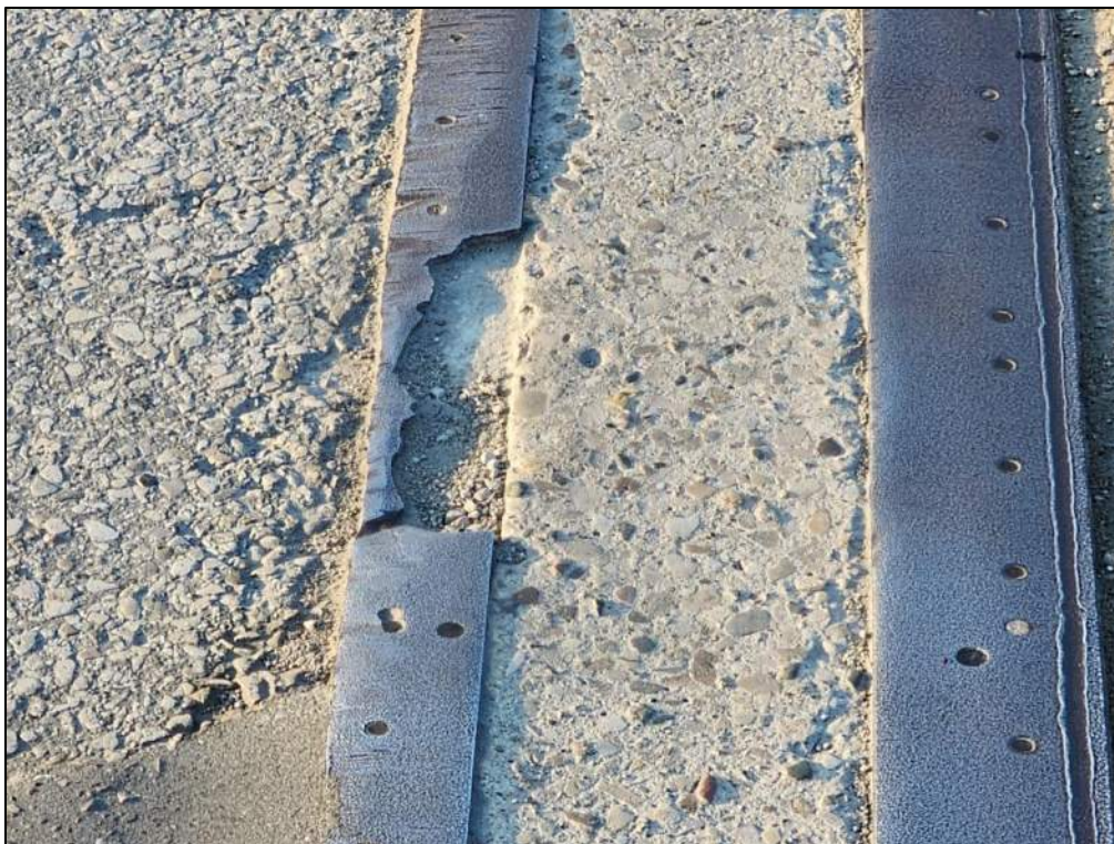
Photo P11 – West Intermediate Expansion Joint (damaged steel armoring angles; seals cracks, spalls and scaling at concrete end dams)
