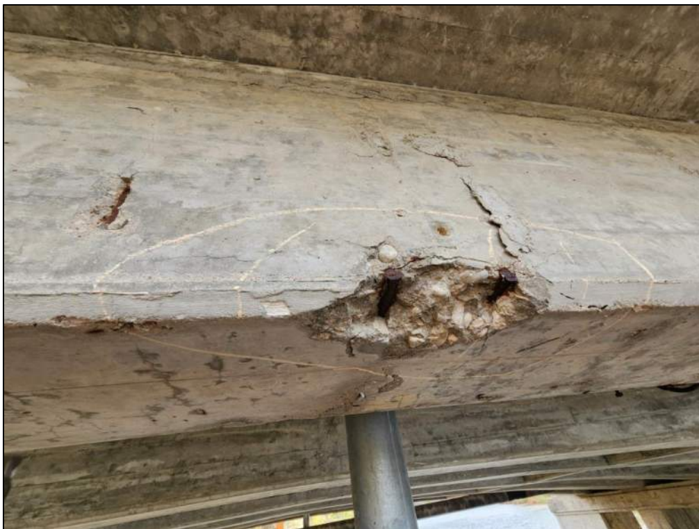
Photo P81 – Girder between Pier 3 and Pier 4 (spall with exposed corroded rebar and delamination)
