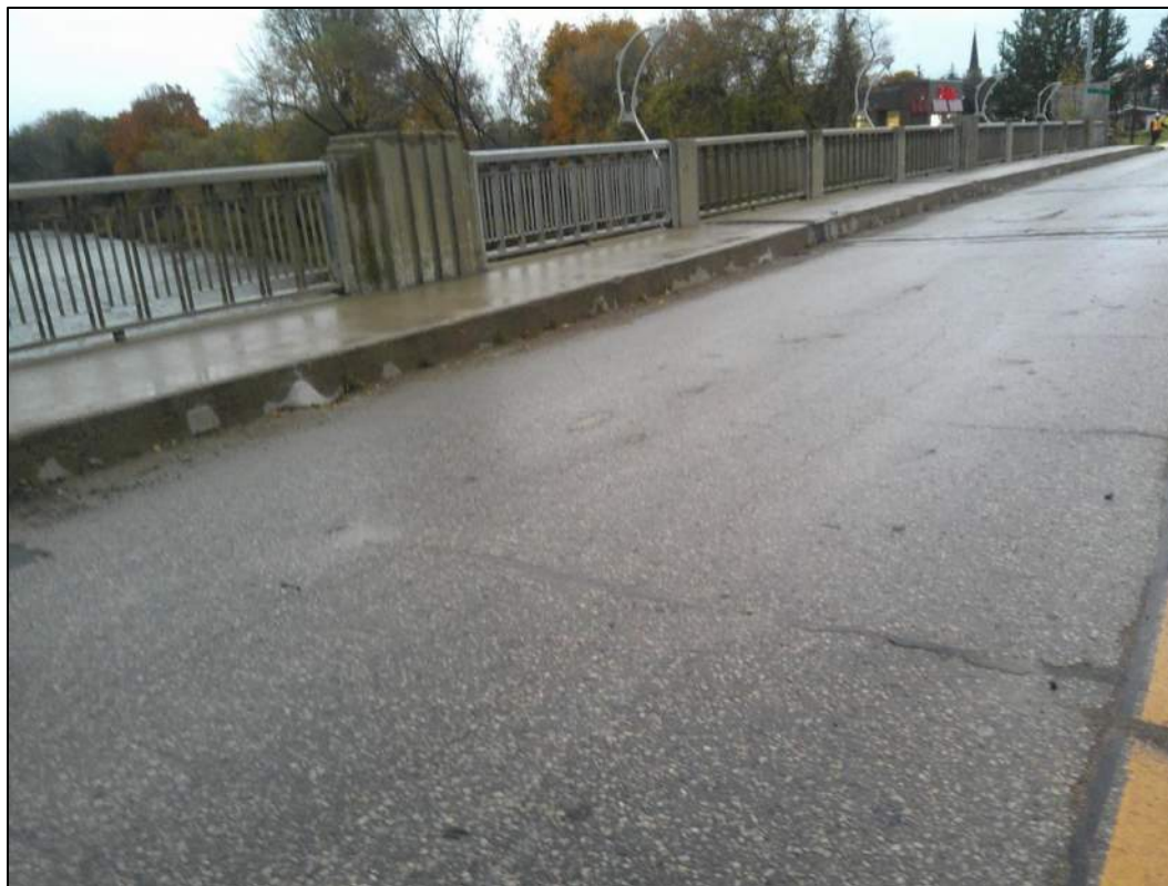
Photo P5 – Asphalt Wearing Surface (good condition – sealed/unsealed cracks, light ravelling, light rutting and patched areas)
