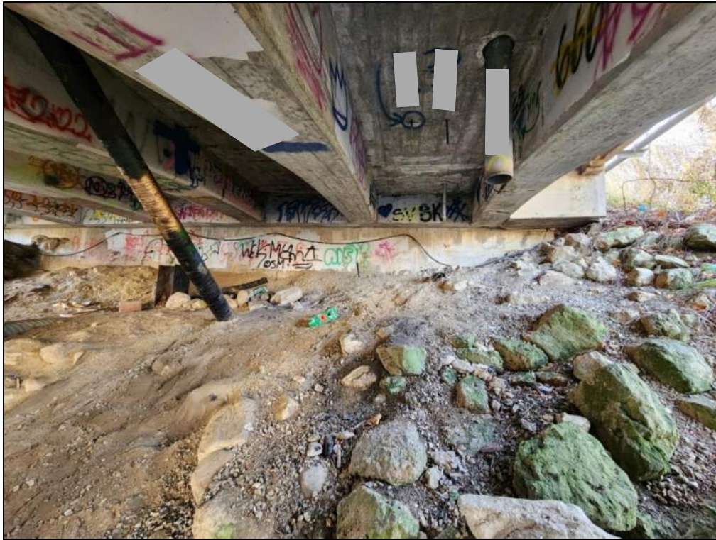
Photo P37 – West Abutment (good condition) and Embankment (fair to good condition – erosion, loss of rock protection)
