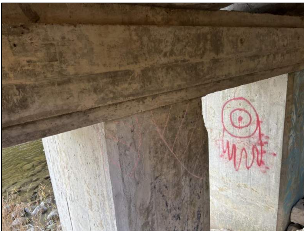
Photo P54 – Pier 4 – East Face (spall and delamination)
