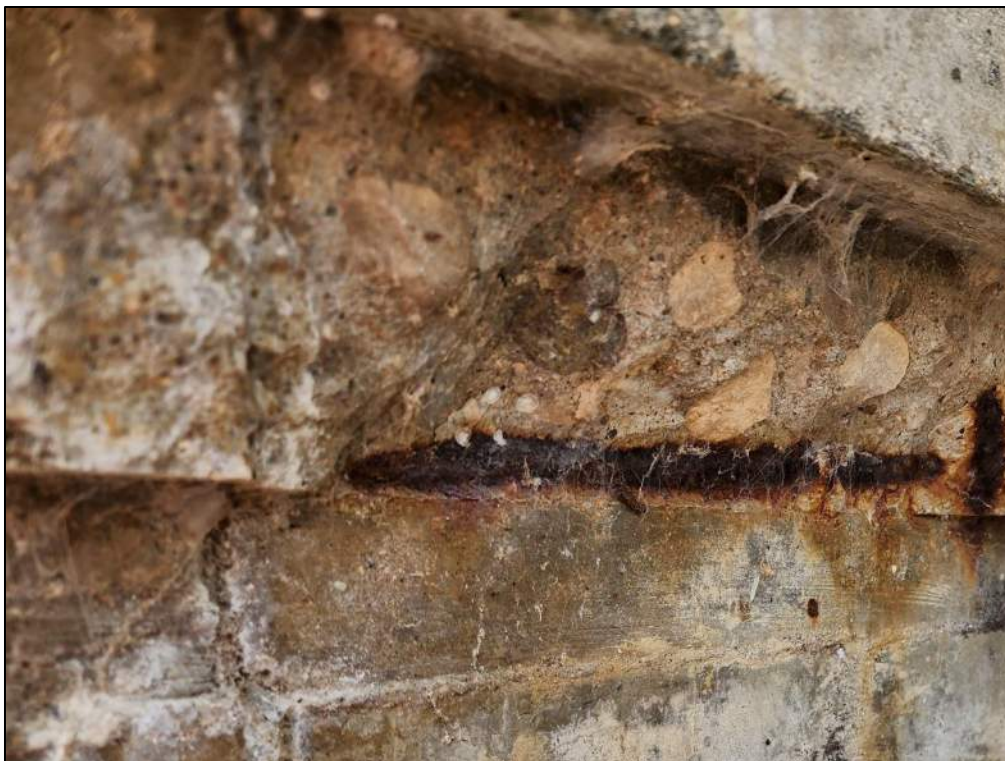
Photo P47 – Pier 2 – East Face (spall with exposed corroded rebar)
