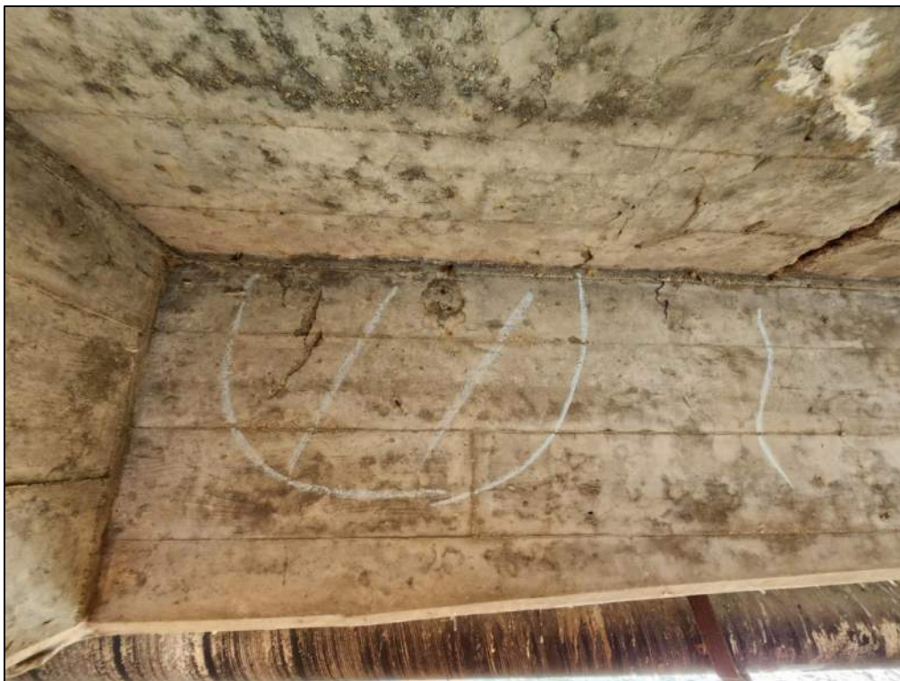
Photo P83 – Girder between Pier 2 and Pier 3 (delamination)
