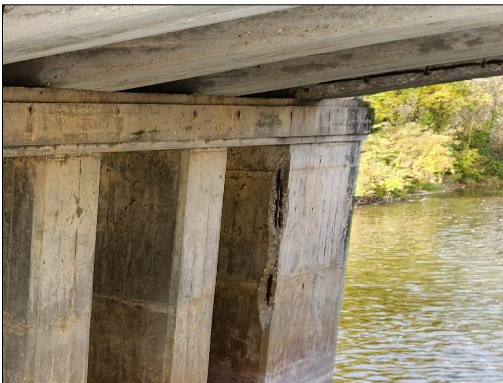
Photo P48 – Pier 2 – East Face (spall with exposed rebar)
