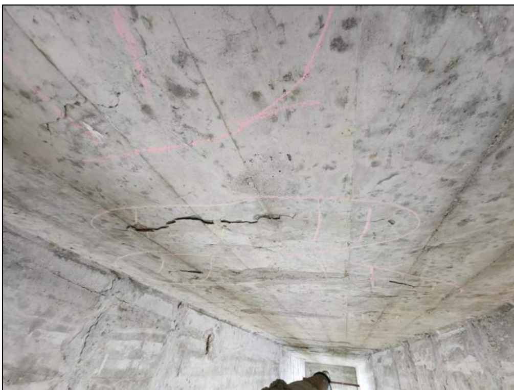
Photo P72 – Soffit between Pier 3 to Pier 4 (spall with exposed corroded rebar, delamination and patched area)
