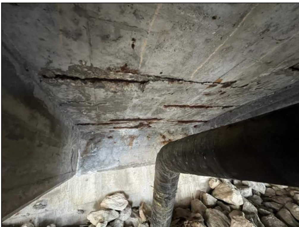
Photo P74 – Soffit between East Abutment to Pier 4 (spall with exposed corroded rebar, delaminations and patched areas)
