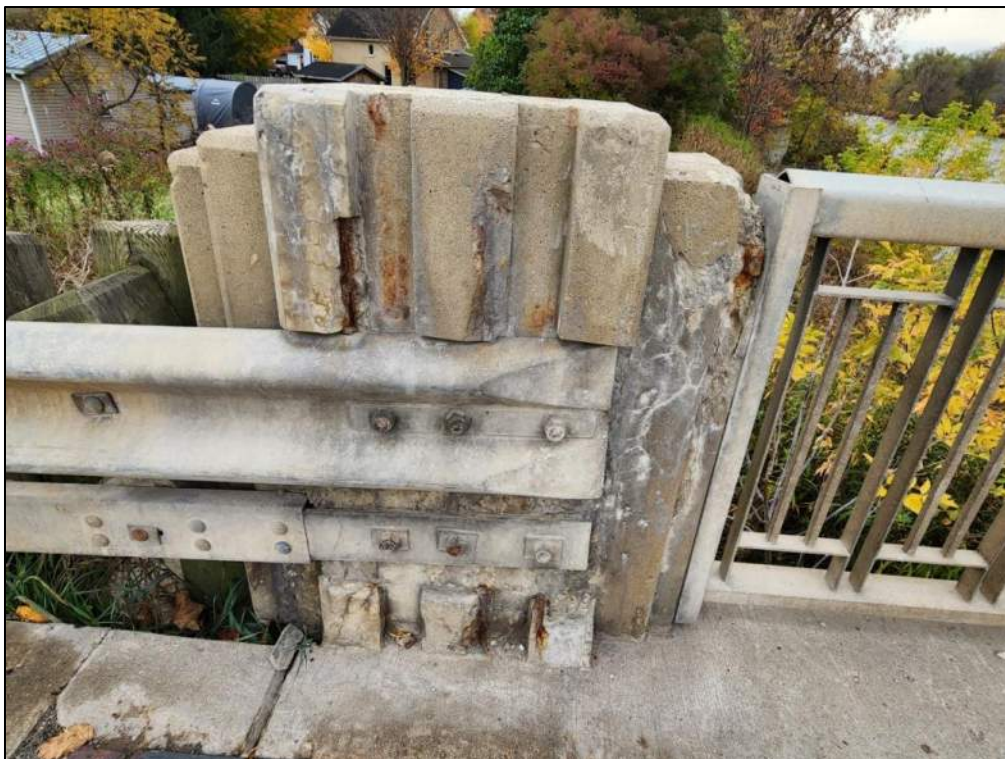
Photo P29 – South-East End post (AAR, spalls with exposed corroded rebar)
