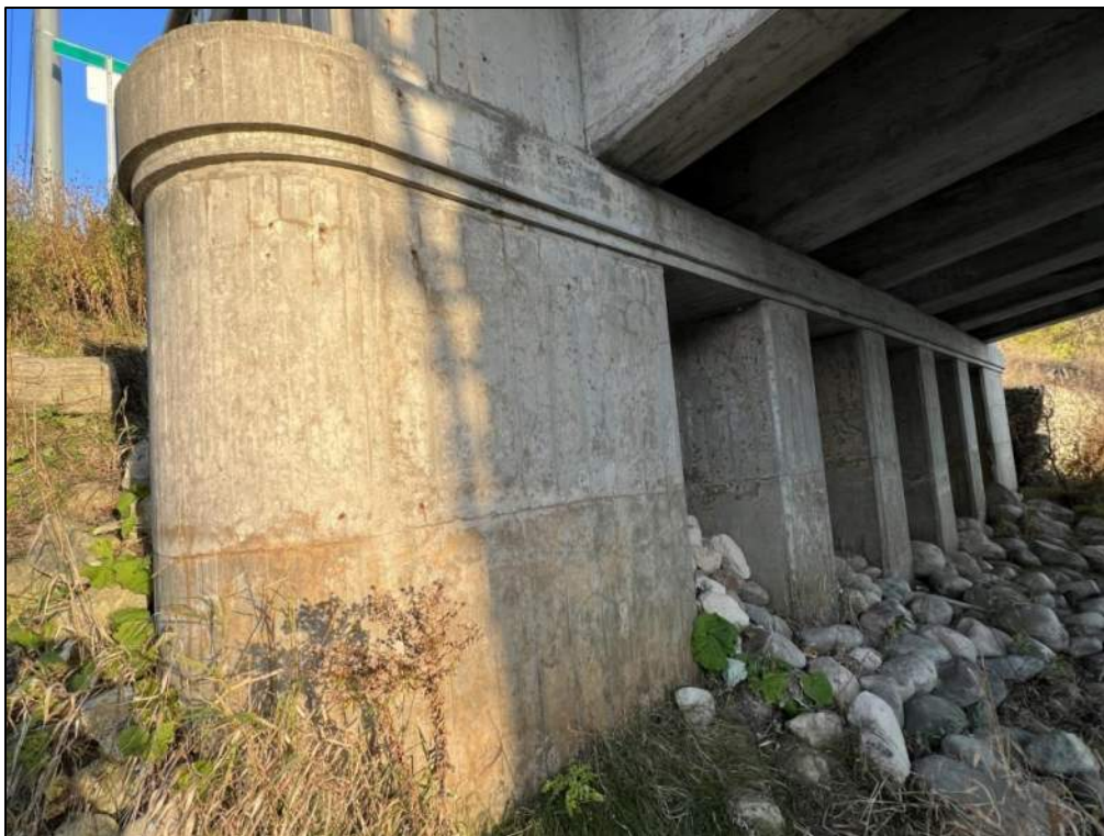
Photo P55 – Pier 4 – West Face (cracks, spall, delamination and light scaling)
