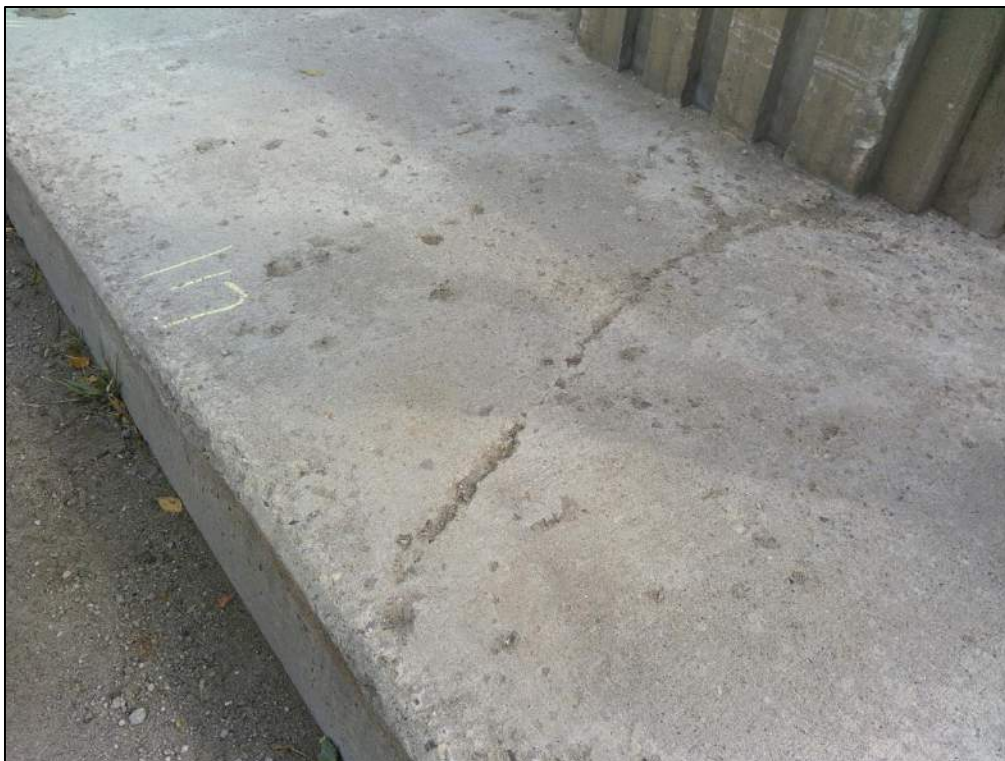
Photo P21 – South Sidewalk (crack above Pier 2, shallow pop-outs – typical)
