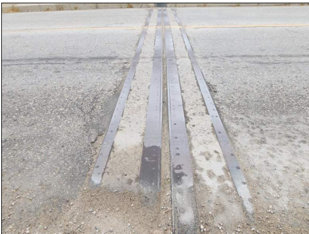
Photo P8 – West Expansion Joint (strip seal joint, light rusting on the steel armoring angles; seals covered with dirt and debris; cracks, spalls and scaling at concrete end dams-gap dimensions vary from 40mm to 45mm)
