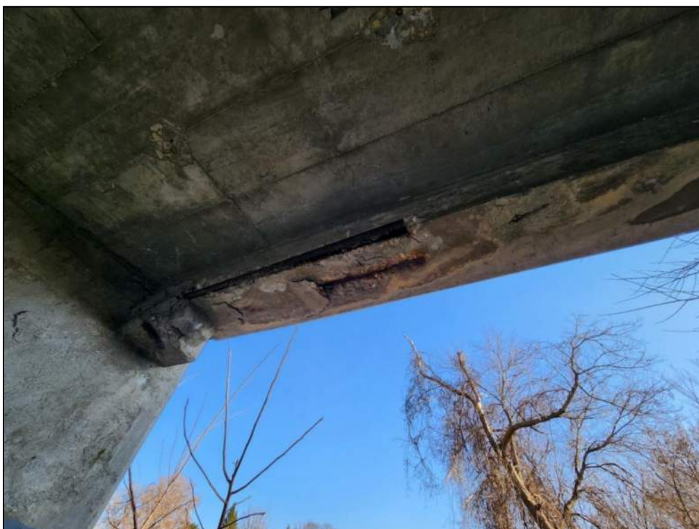
Photo P58 – Girder between West Abutment and Pier 1 (spall with exposed corroded rebar)
