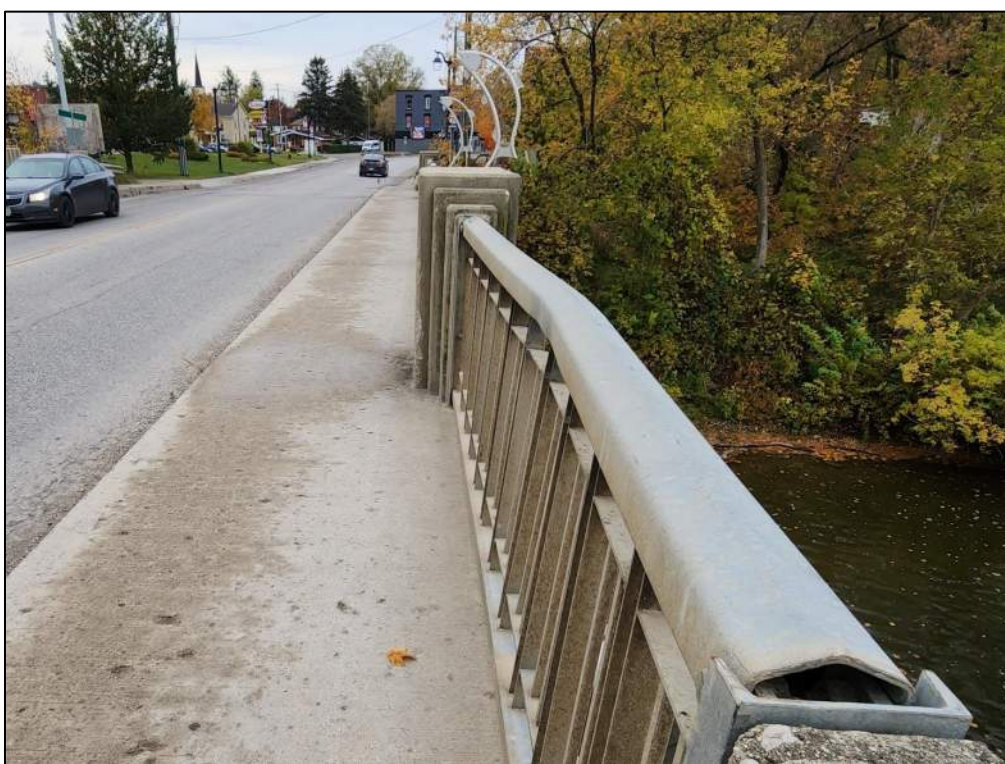
Photo P18 – North Steel Handrail (impact damage, bent railings) and Sidewalk (pop-outs)
