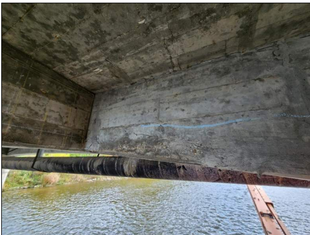
Photo P80 – Girder between Pier 2 and Pier 3 (delamination)
