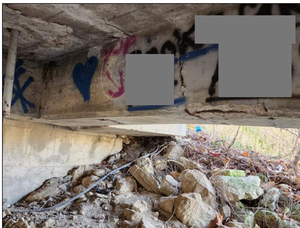
Photo P76 – Girder between West Abutment and Pier 1 (cracks, spall with exposed corroded rebar, delamination)
