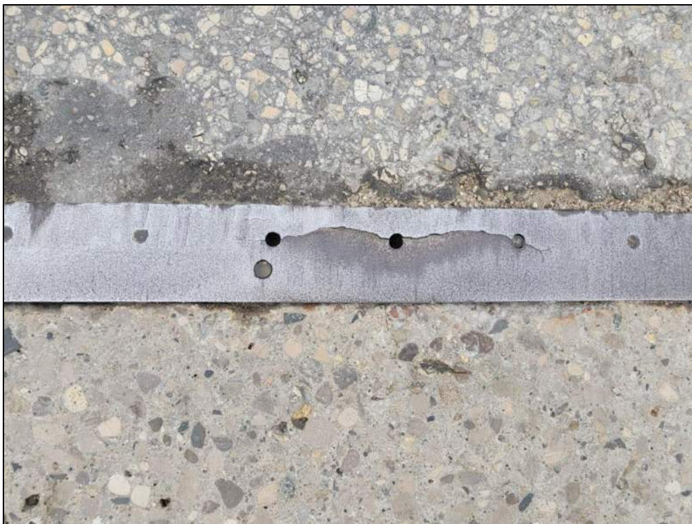
Photo P13 – East Expansion Joint (cracks on the steel armoring angles; cracks, spalls and scaling at concrete end dams)
