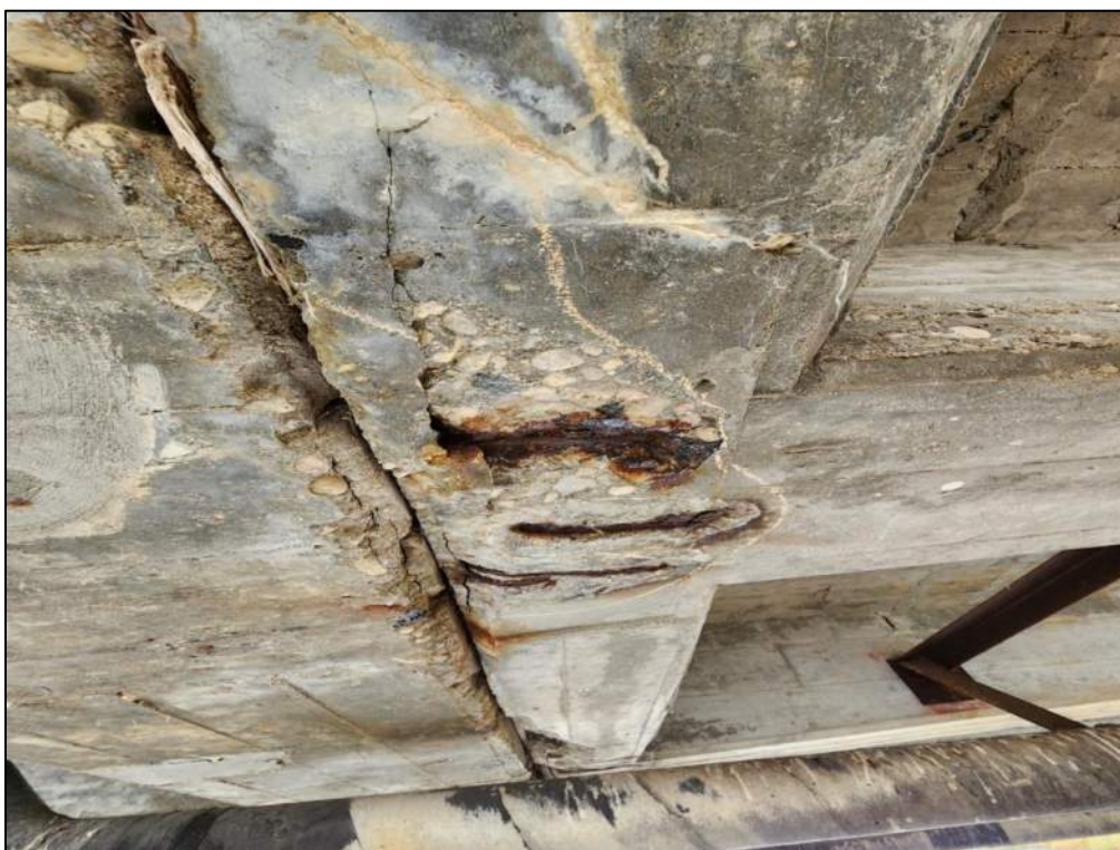
Photo P66 – Soffit between Pier 2 to Pier 3 (spall with exposed corroded rebar and delamination at bottom face of diaphragm; evidence of leakage)
