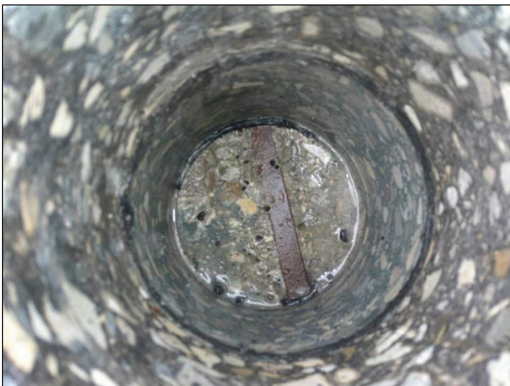
Photo P92 – Inside Core C3 (square rebar-light rust)
