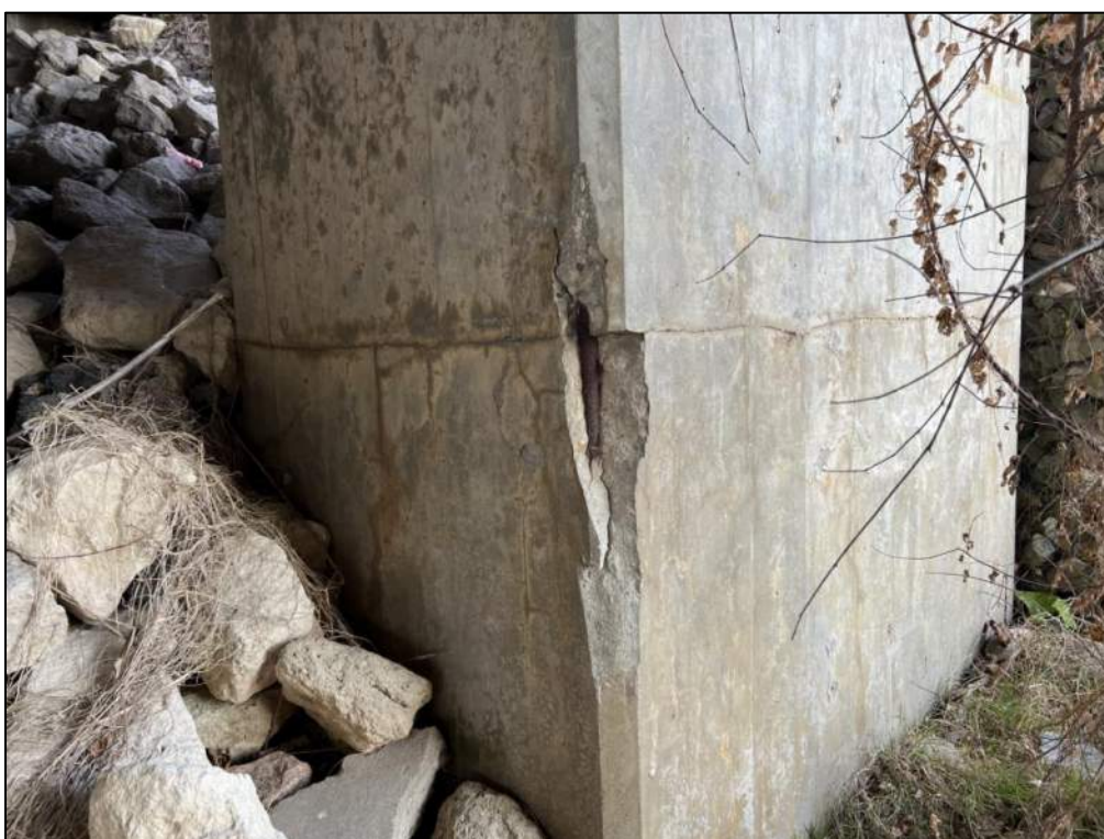
Photo P56 – Pier 4 – West Face (spall, delamination, and light scaling)
