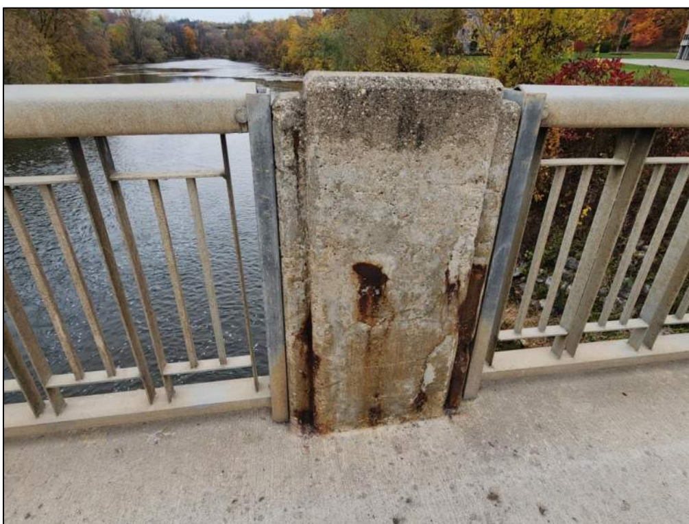
Photo P26 – North Concrete Post (severe rust stains)
