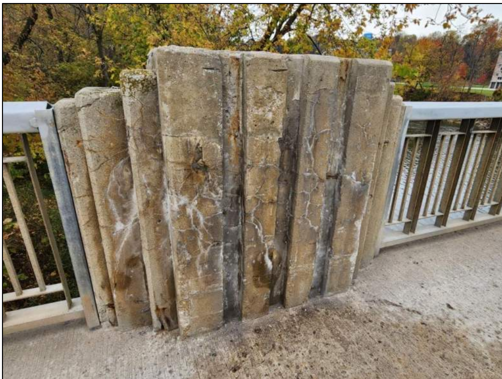
Photo P25 – North Concrete Post (severe AAR, cracks)
