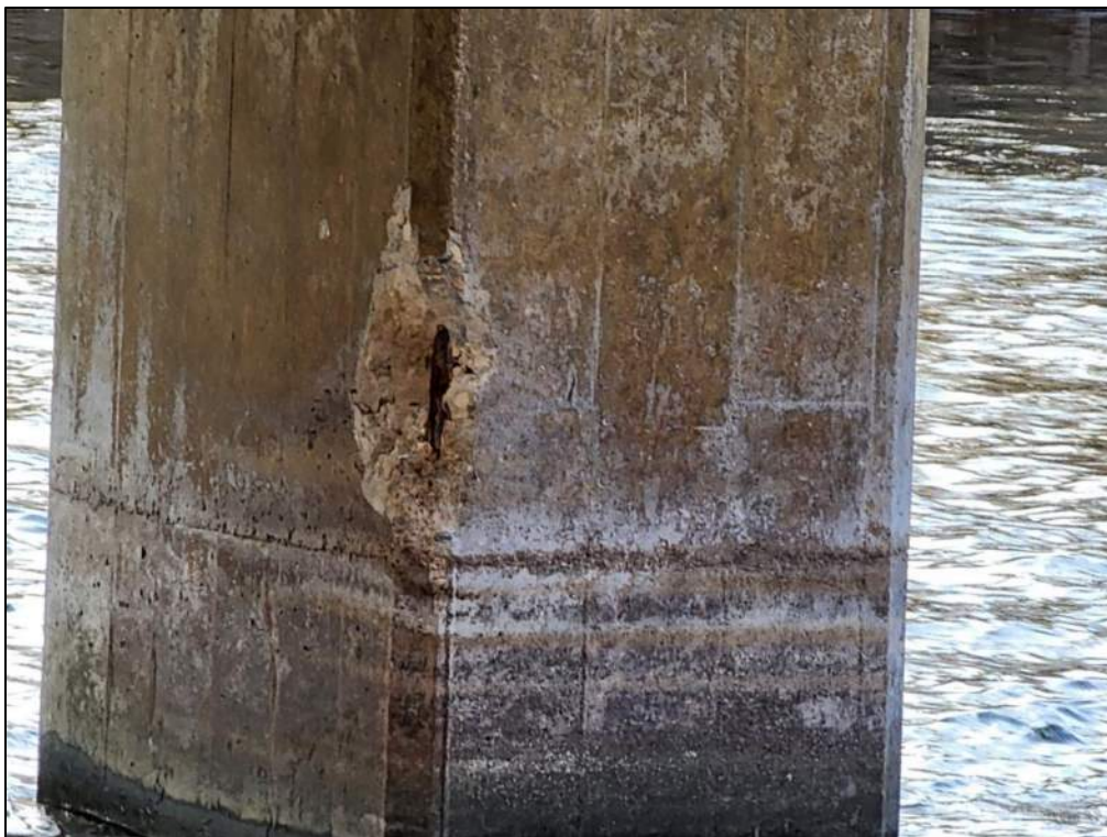
Photo P53 – Pier 3 – East Face (spall with exposed corroded rebar and light scaling)
