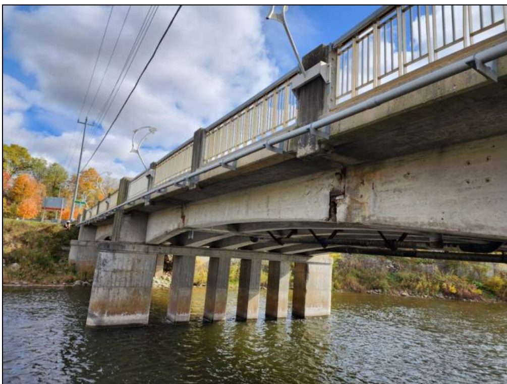
Photo P62 – Soffit between Pier 2 to Pier 3 (spall with exposed rebar, delamination and patched area) and Girder (delamination and patched area)
