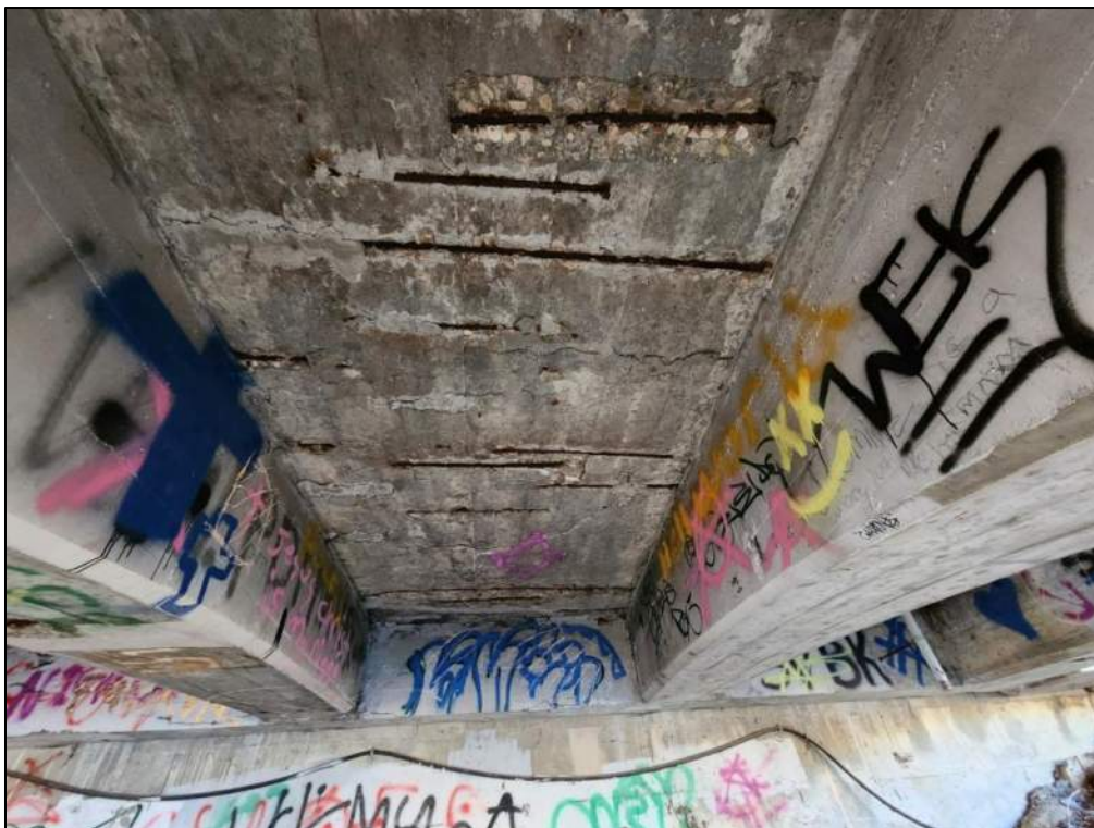
Photo P57 – Soffit between West Abutment and Pier 1 (poor condition – cracks, spall with exposed corroded rebar, delaminations and patched areas)
