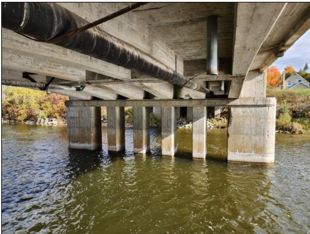
Photo P49 – Pier 3 – West Face (cracks, spall with exposed corroded rebar and delamination and light pattern cracks)
