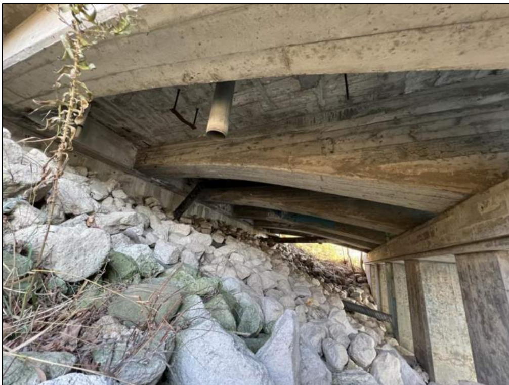
Photo P73 – Soffit between East Abutment to Pier 4 (spall with exposed corroded rebar, delaminations and patched areas) and Girder (delaminations and patched areas)
