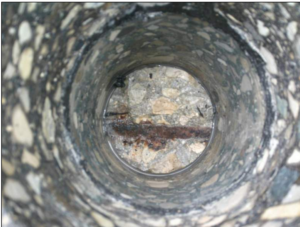
Photo P93 – Inside Core C4 (square rebar-severe rust)
