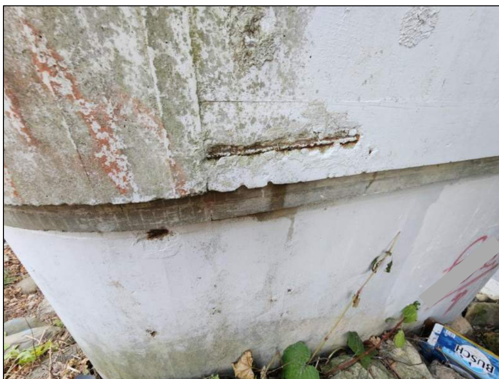
Photo P40 – Pier 1 – West Face (exposed corroded rebar)
