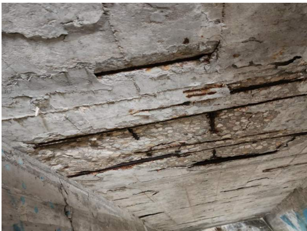
Photo P75 – Soffit between East Abutment to Pier 4 (spalls with exposed corroded rebar, delaminations and patched areas)
