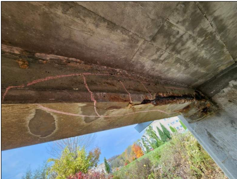
Photo P70 – Girder between Pier 3 to Pier 4 (spall with exposed corroded rebar, delamination and patched area)
