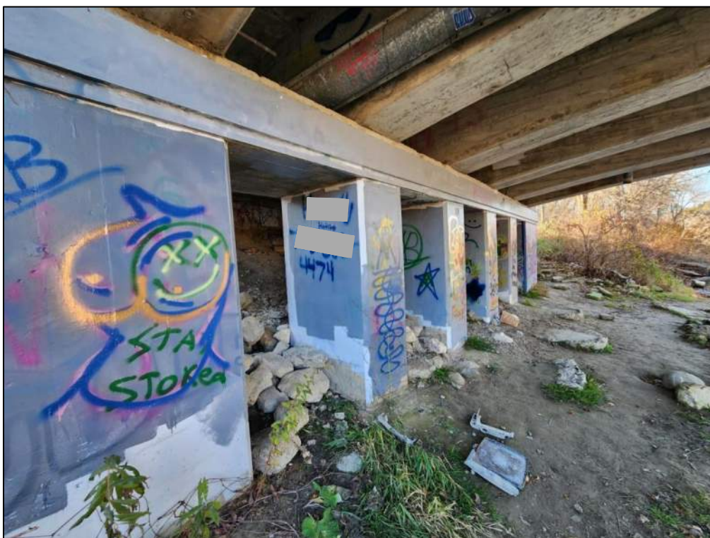
Photo P42 – Pier 1 – East Face (cracks, spall and exposed rebar)
