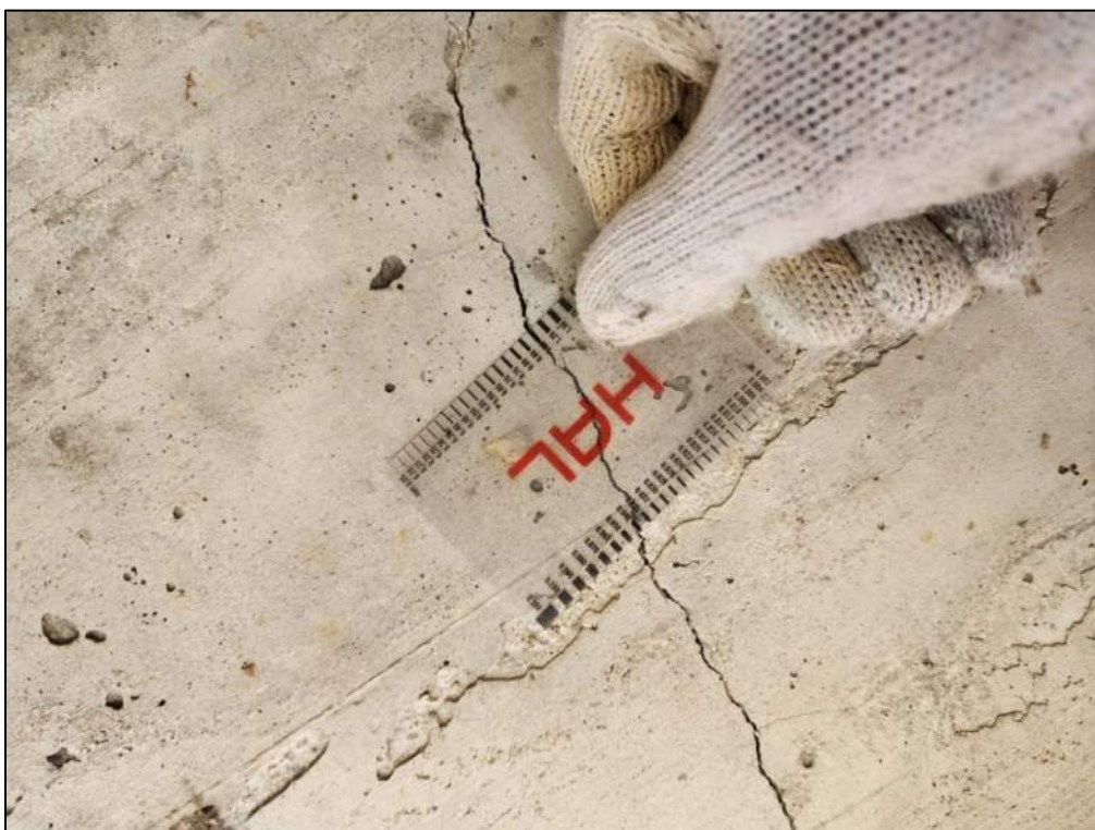
Photo P82 – Girder between Pier 3 and Pier 4 (wide crack)
