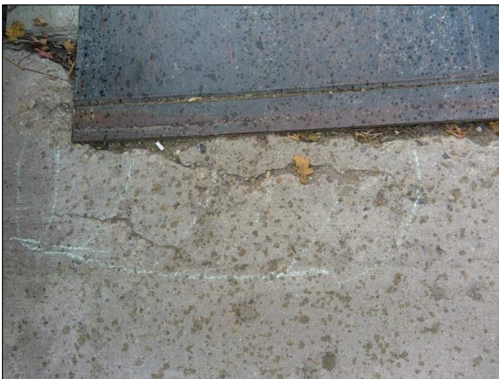
Photo P22 – South Sidewalk (crack and delamination)
