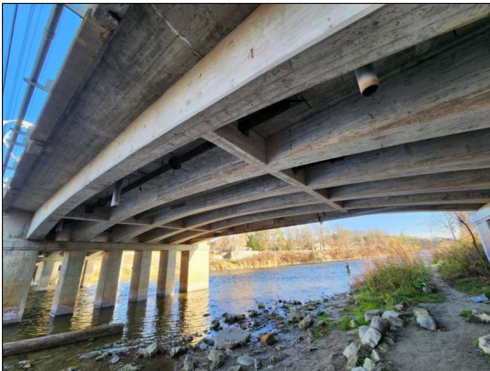
Photo P59 – Soffit between Pier 1 to Pier 2 (cracks, spall with exposed corroded rebar, delaminations and patched areas)
