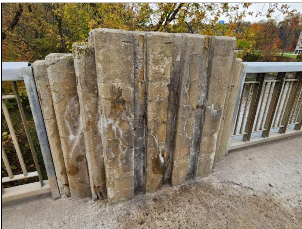
Photo P28 – North-West End post (severe AAR, cracks)
