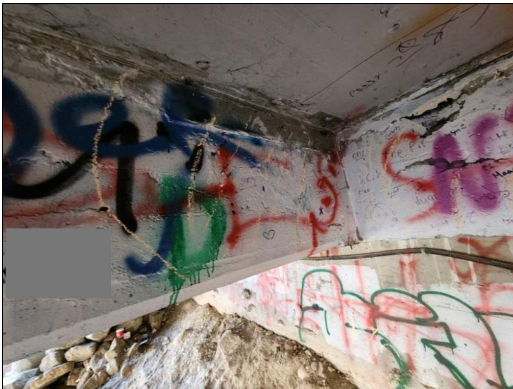
Photo P77 – Girder at West Abutment (delamination)
