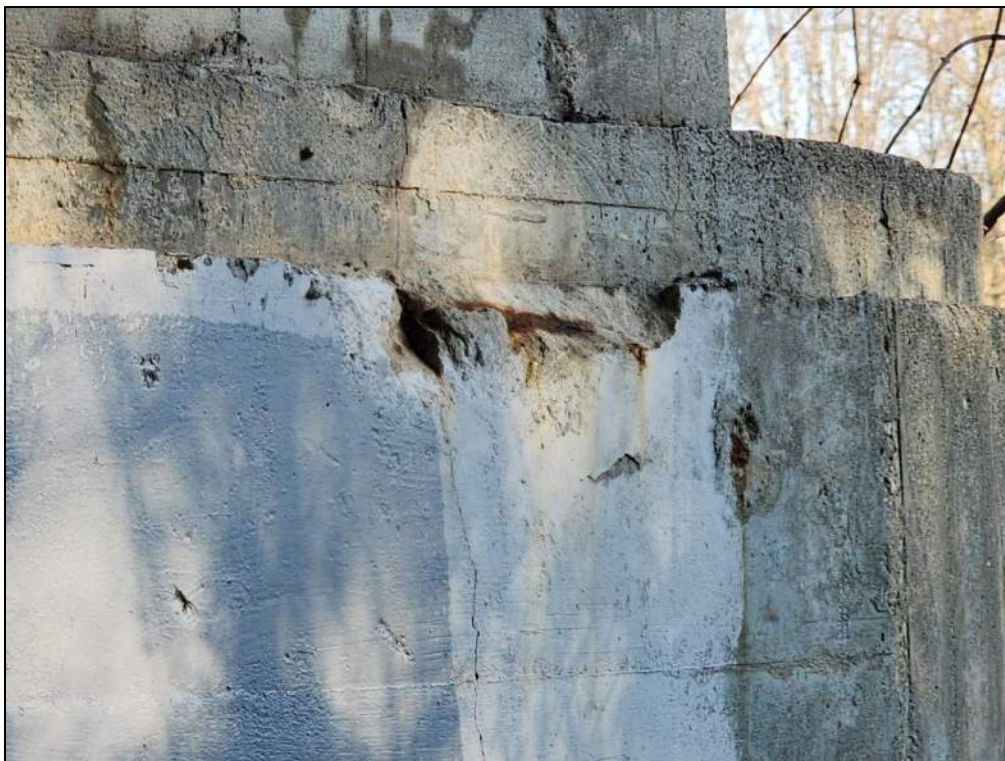
Photo P41 – Pier 1 – West Face (crack, spall with exposed corroded rebar)
