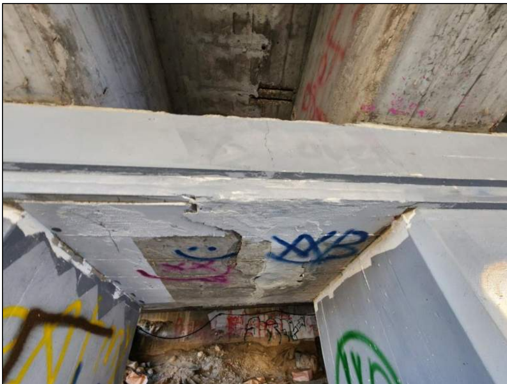
Photo P43 – Pier 1 – East Face (cracks, delamination at bottom face)
