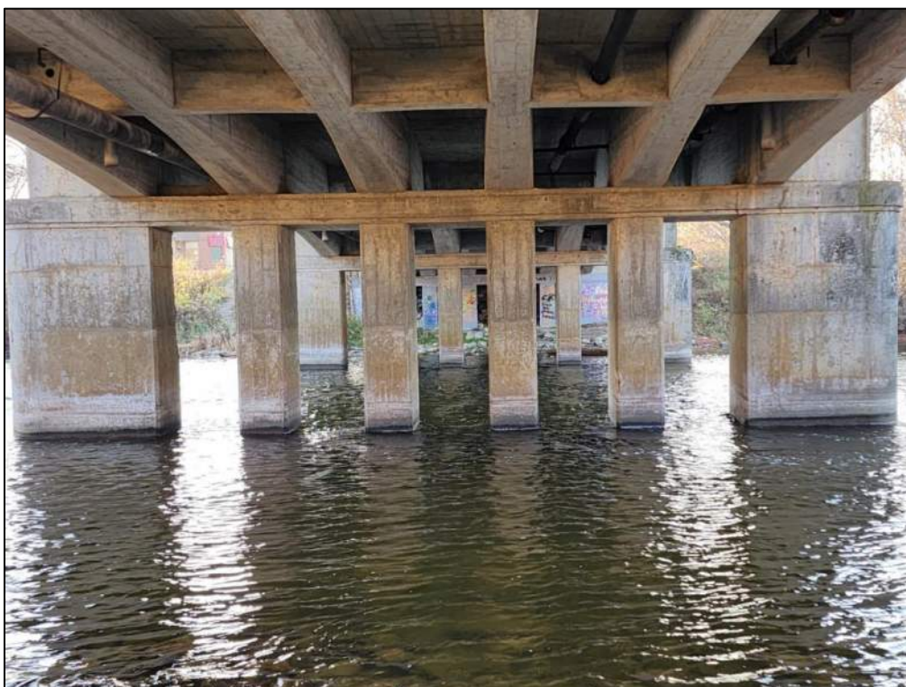
Photo P52 – Pier 3 – East Face (light pattern cracks, spall and light scaling)
