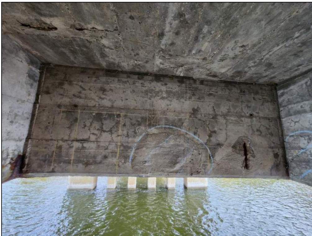
Photo P87 – Diaphragm Between Pier 2 to Pier 3 (spall with exposed corroded rebar and delamination)
