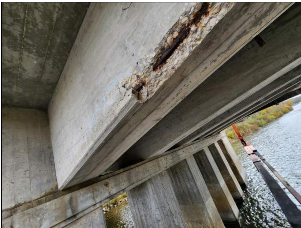
Photo P79 – Girder between Pier 2 and Pier 3 (spall with exposed corroded rebar, delamination)
