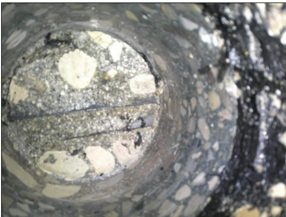
Photo P94 – Inside Core C10 (debonded overlay; square rebar-good condition)
