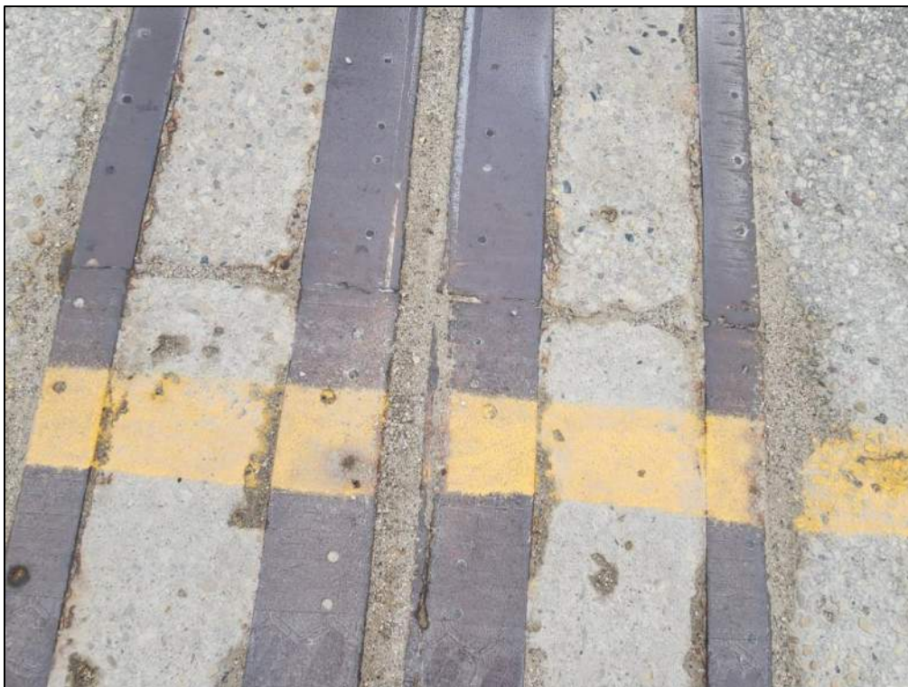
Photo P9 – West Expansion Joint (light rusting on the steel armoring angles; seals covered with dirt and debris; cracks, spalls and scaling at concrete end dams)
