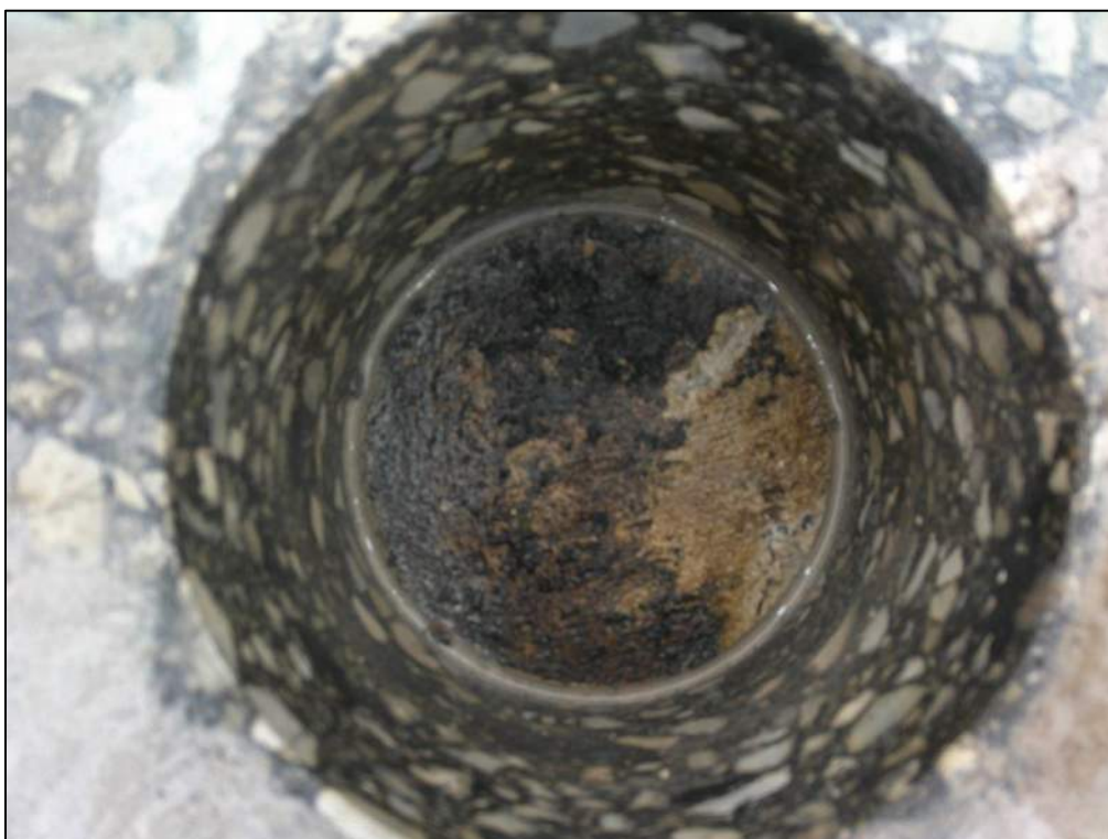
Photo P96 – Inside Core C1 at East Approach (concrete approach slab present)
