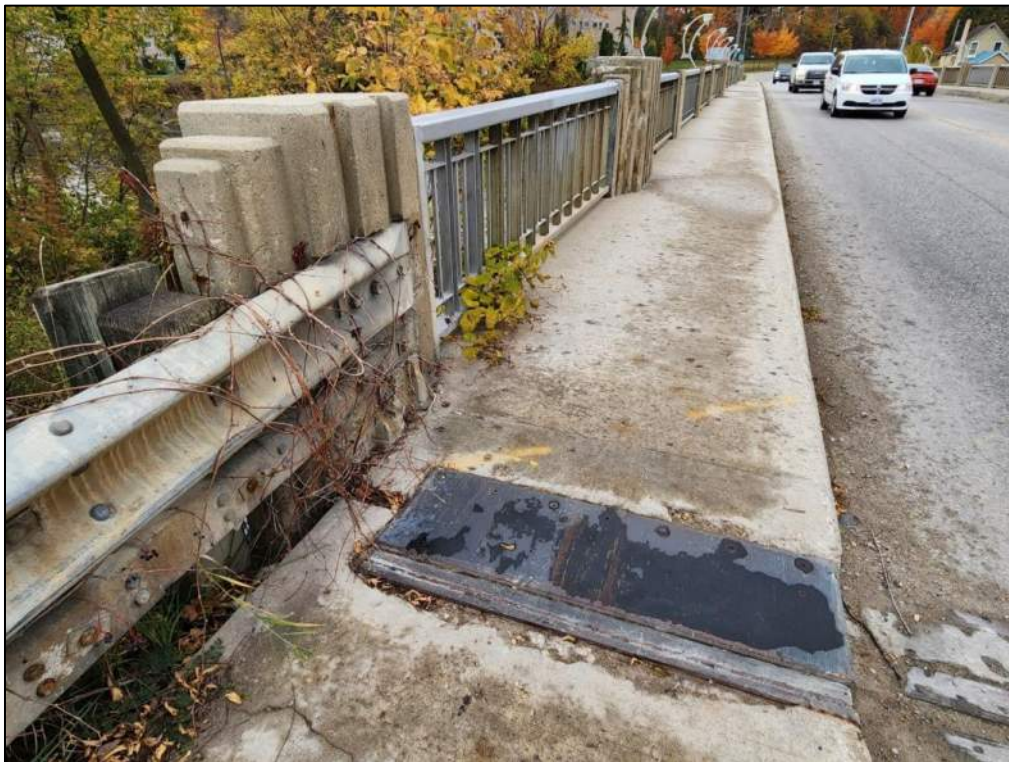
Photo P16 – North Sidewalk (good condition – crack, spalls delamination and shallow pop-outs) and Steel Handrail (fair to good condition – impact damage)
