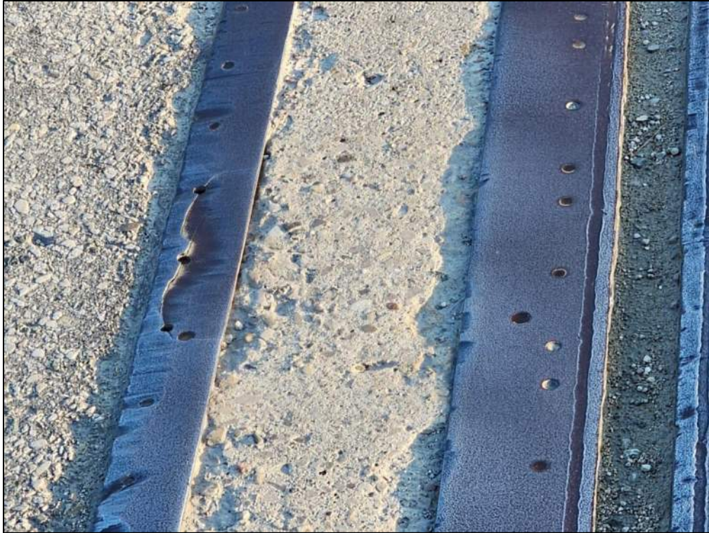
Photo P15 – East Intermediate Expansion Joint (damaged steel armoring angles; seals covered with dirt and debris; cracks, spalls and scaling at concrete end dams)
