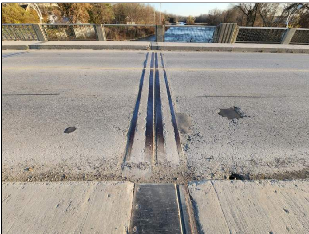
Photo P10 – West Intermediate Expansion Joint (strip seal joint, light rusting on the steel armoring angles; seals covered with dirt and debris; cracks, spalls -gap dimensions are 50mm at north corner and 55mm at centre and south cor gap dimensions vary from 50mm to 55mm)
