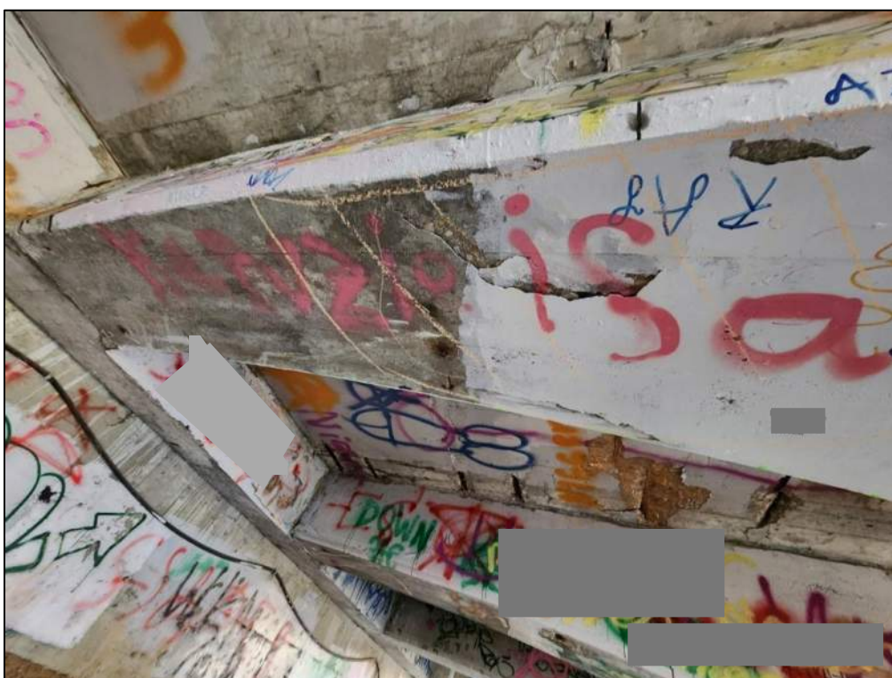
Photo P78 – Girder between West Abutment and Pier 1 (delamination)
