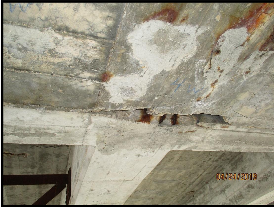
Typical pop-outs, corner spall from insufficient cover
